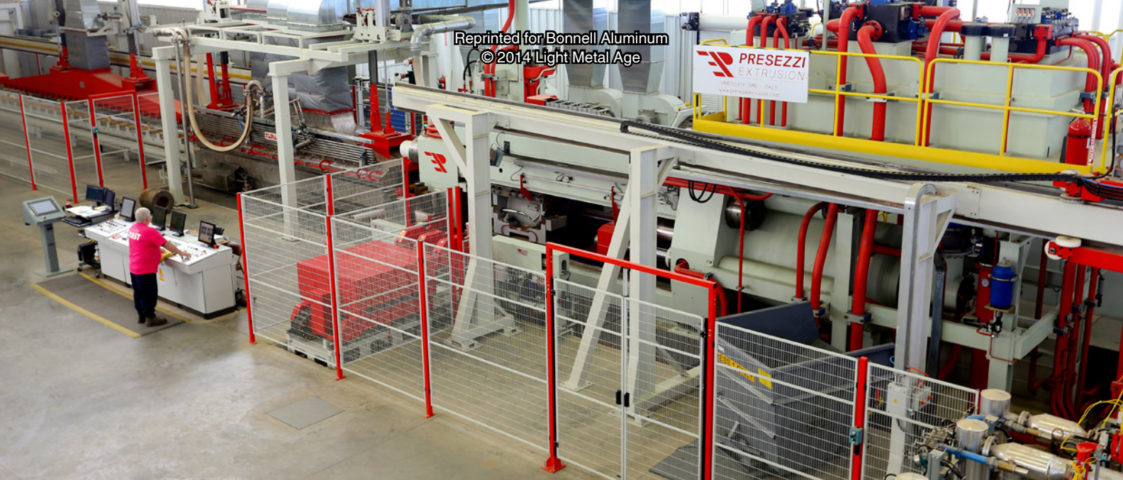
The new 3,600 ton, 9 inch press installed at Bonnell's Newnan facility is dedicated to automotive production.
